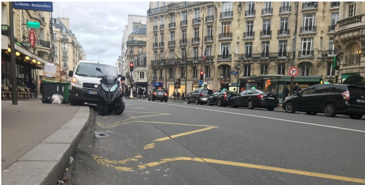
Figure 20. Road surface damage and illegal parking at a bus stop
